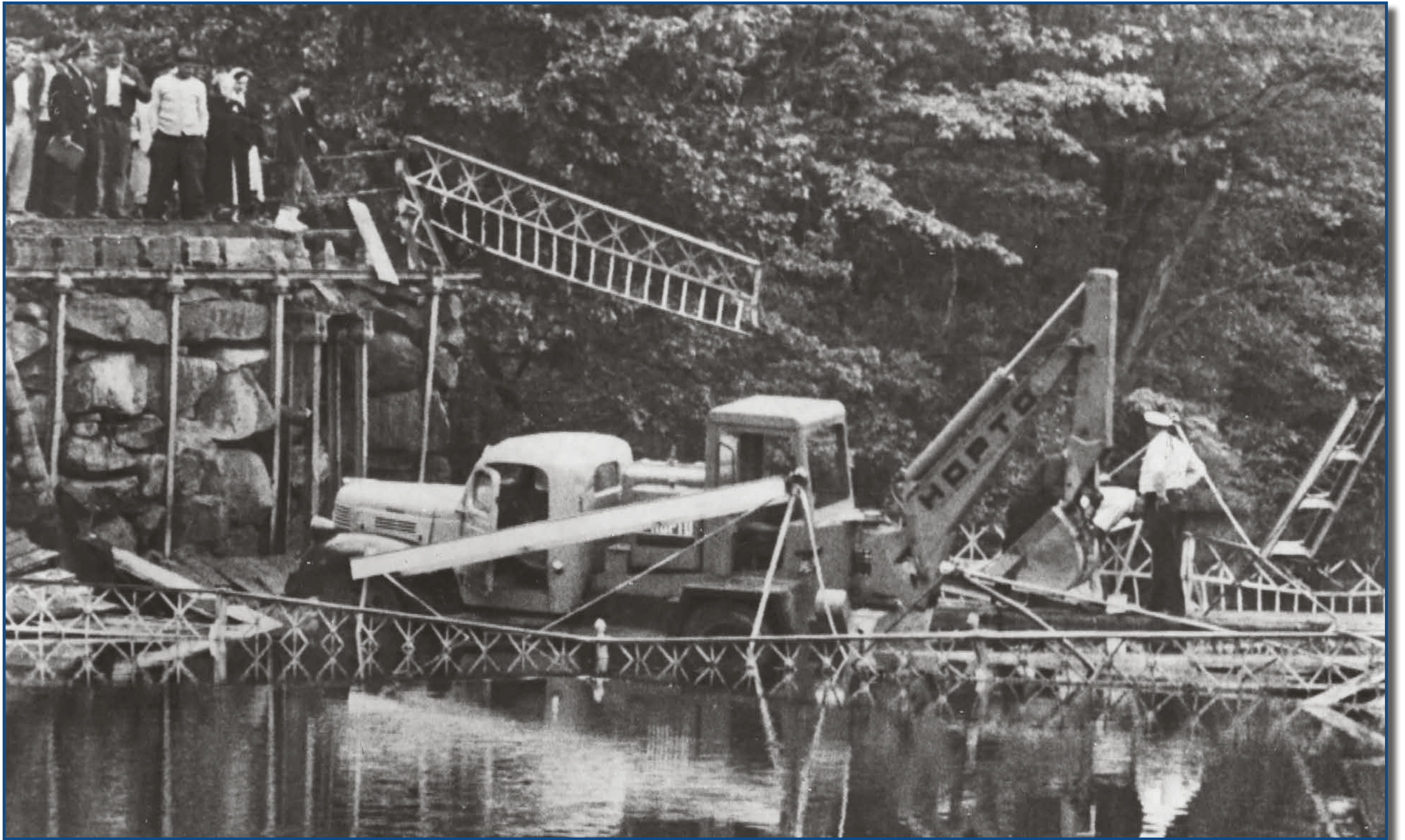
Truck mounted Hopto backhoe collapses bridge over Beaver Brook, Dracut, 1956
